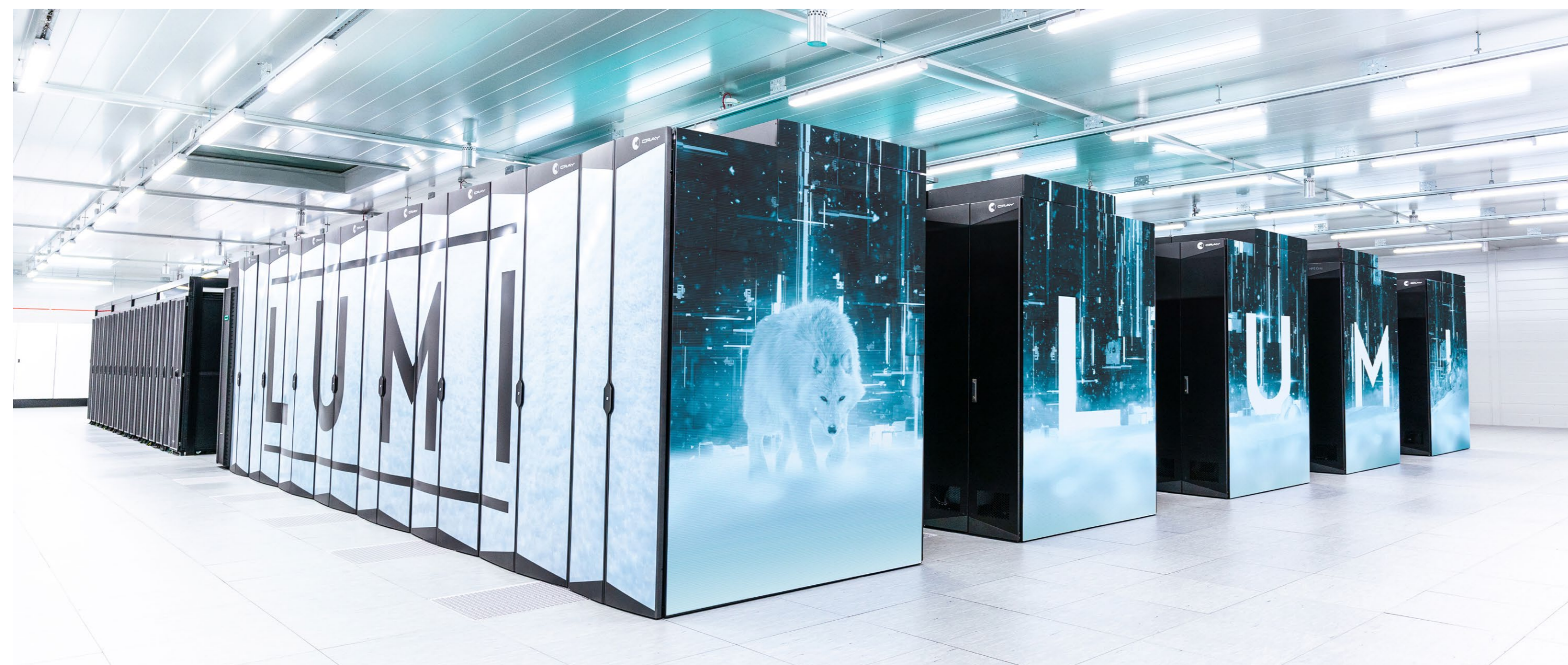
Figure 1. Cabinets of the LUMI supercomputer.
